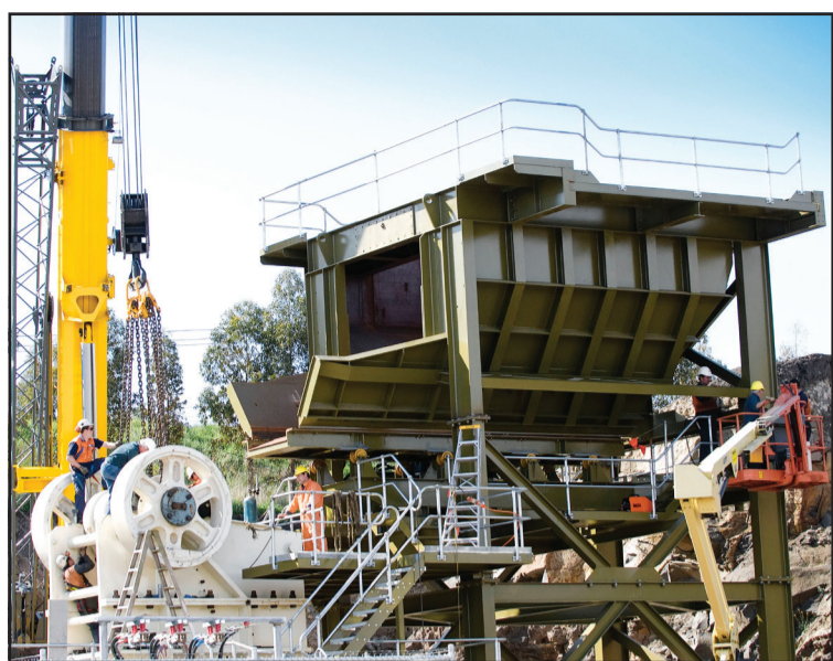
Photo 4 Northern Quarries primary crushing station
